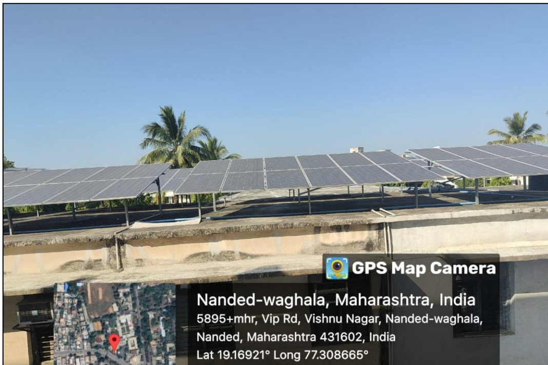
Photograph of Roof Top Solar PV Plant:
